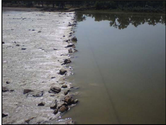
Intake Diversion Dam is listed as a probable source of impairment related to fish passage. Flow is 2,000 cfs in this photograph.
