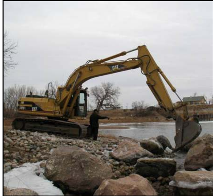
Construction of a rock ramp near Miles City, Montana (photo courtesy of FWP)
