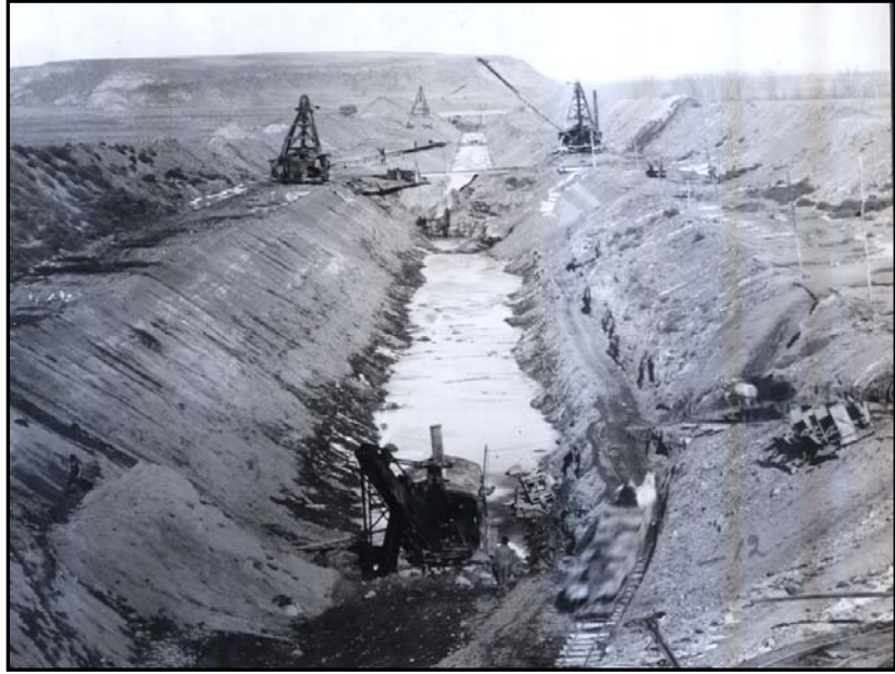
Construction of the main canal just below the intake gates in November 27, 1908
